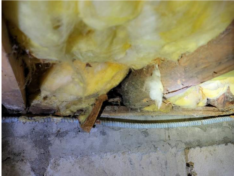
Deterioration of sill and joist.
