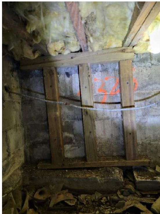
Typical previous repair.
