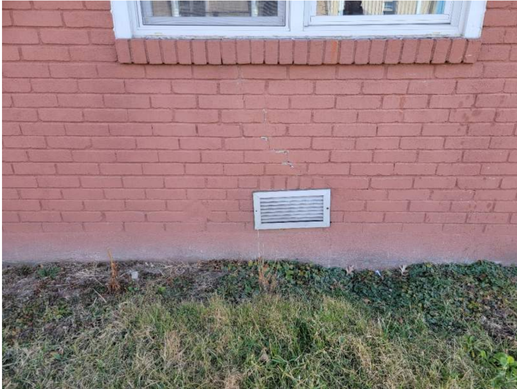
Recent crack above air vent.
