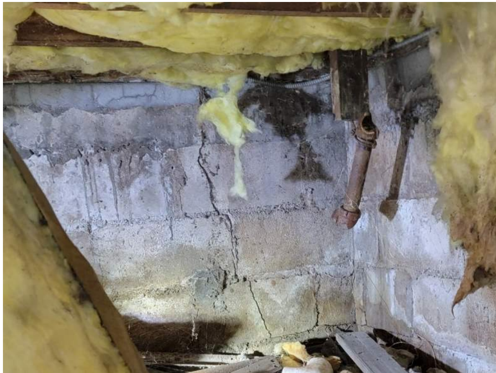
Typical crack in masonry foundation wall.
