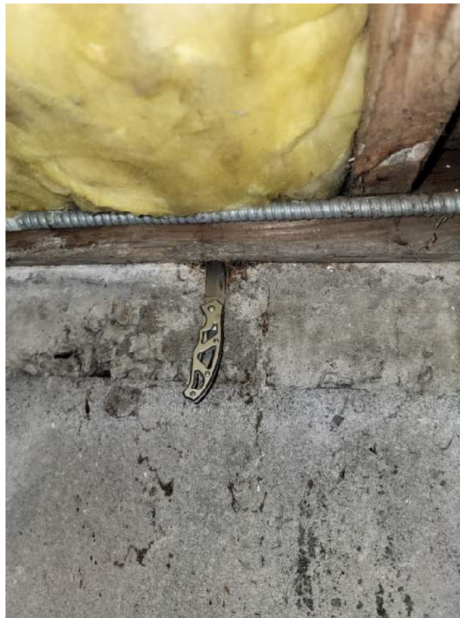
Deterioration of sill and joist.
