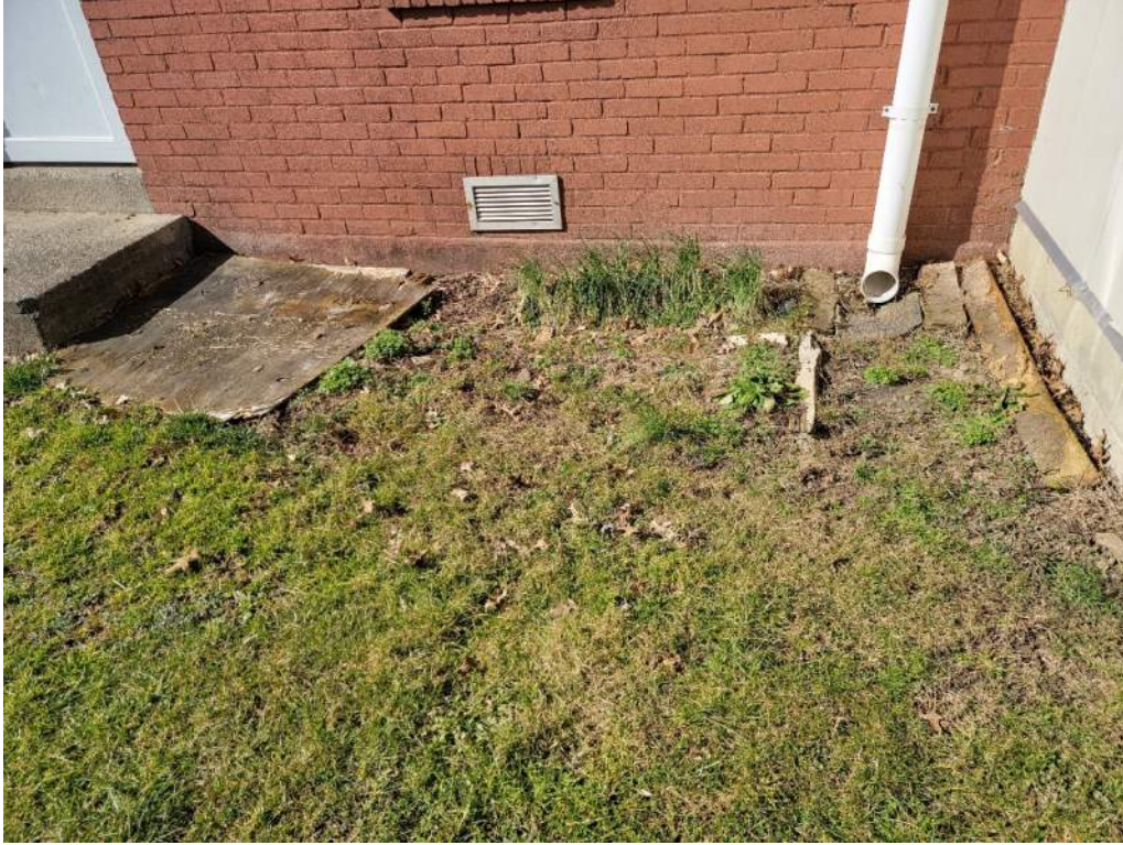
Earth grades flowing back towards foundation wall.
