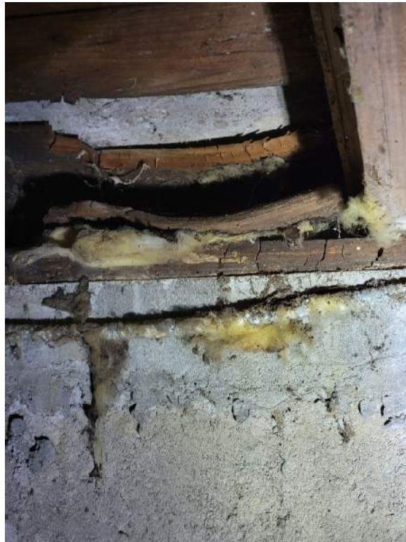
Laundry room floor deterioration and concrete slab.
