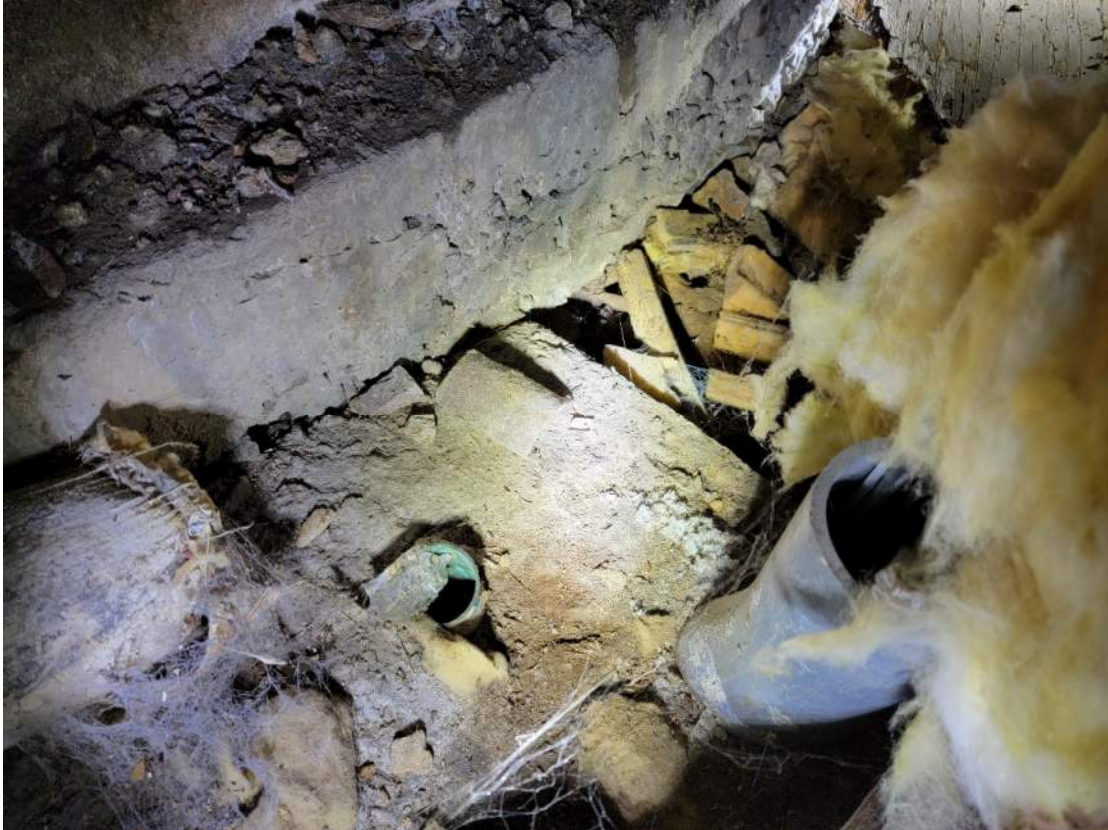
Undermined wall footing.
