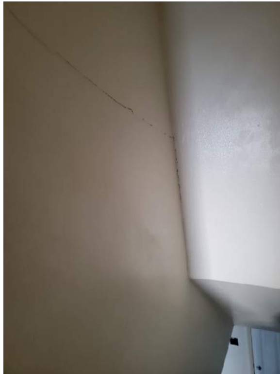
Typical crack in stair well.
