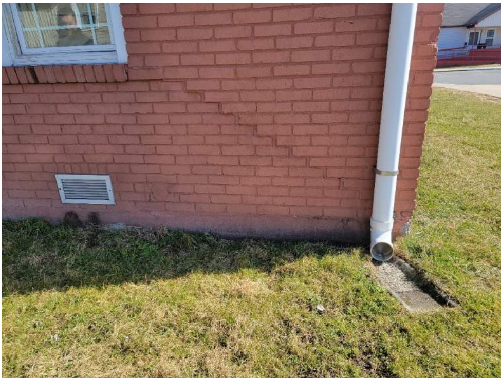
Typical historic rack and lateral displacement.
