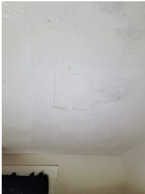
Typical ceiling crack in bedroom.
