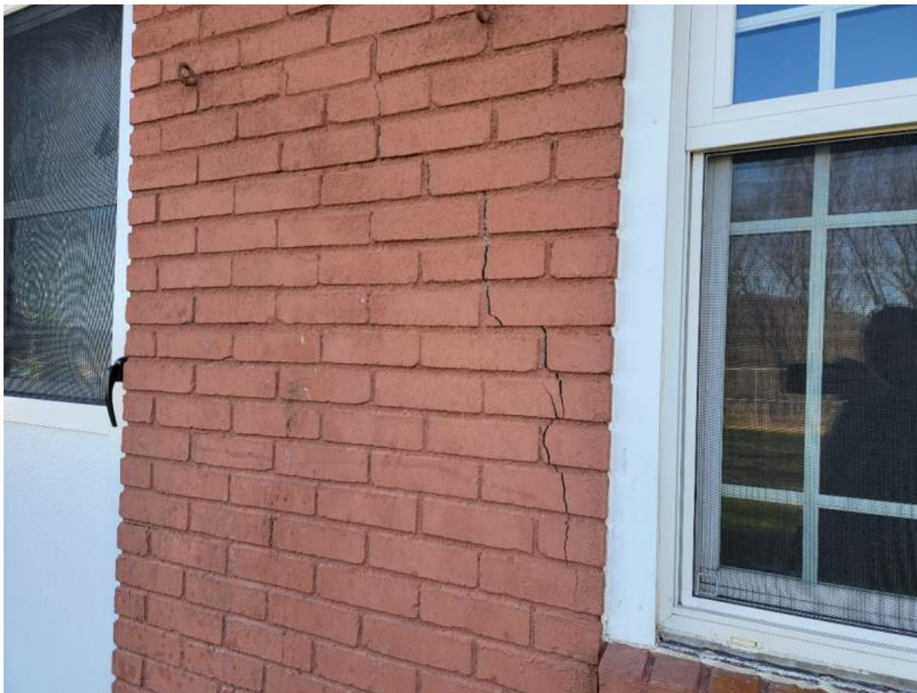
Recent wider crack..
