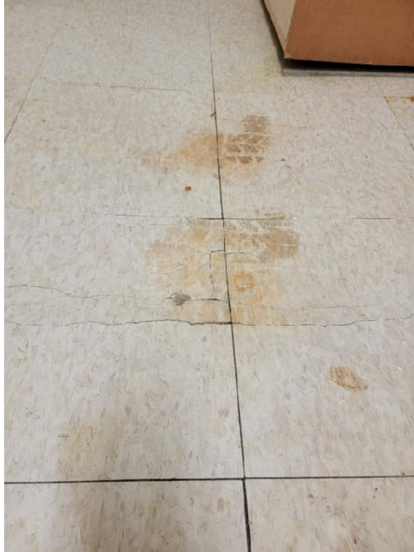
Laundry room floor deterioration.
