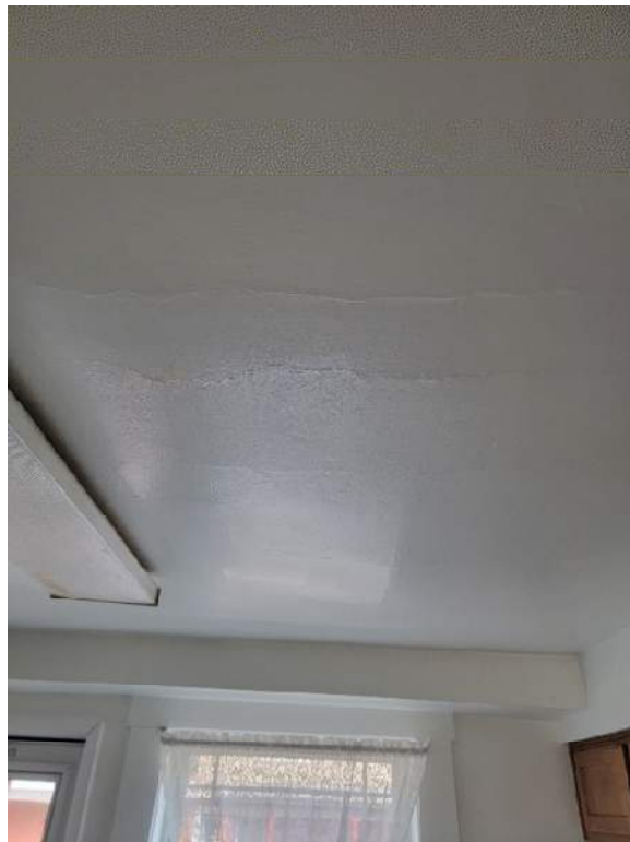
Typical ceiling crack in kitchen.
