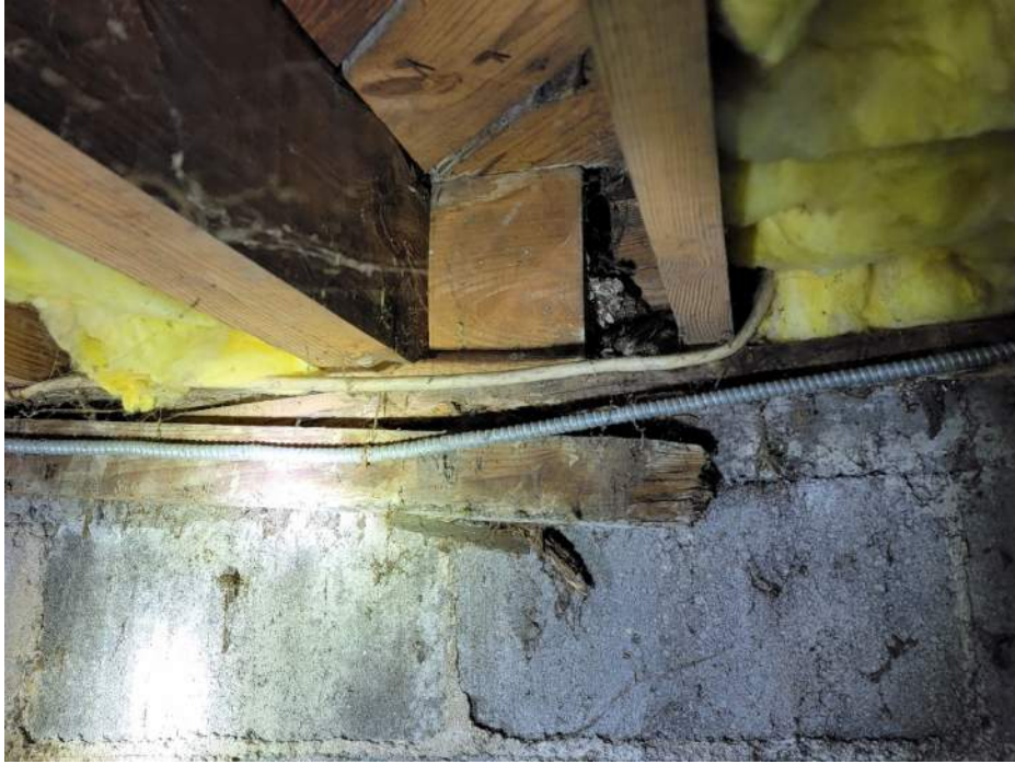
Failing ledger board.
