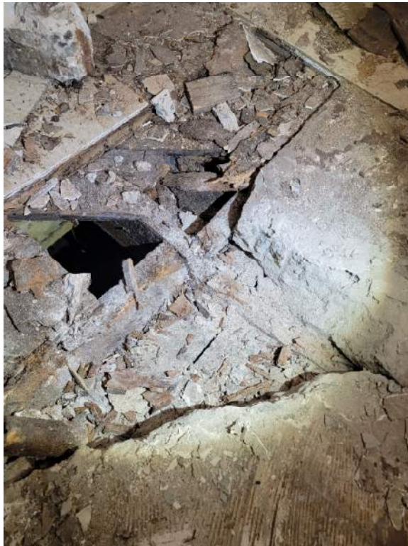
Laundry room floor finish removed showing deterioration and top of concrete slab.
