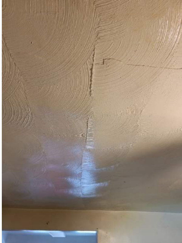
Typical ceiling crack in living room.
