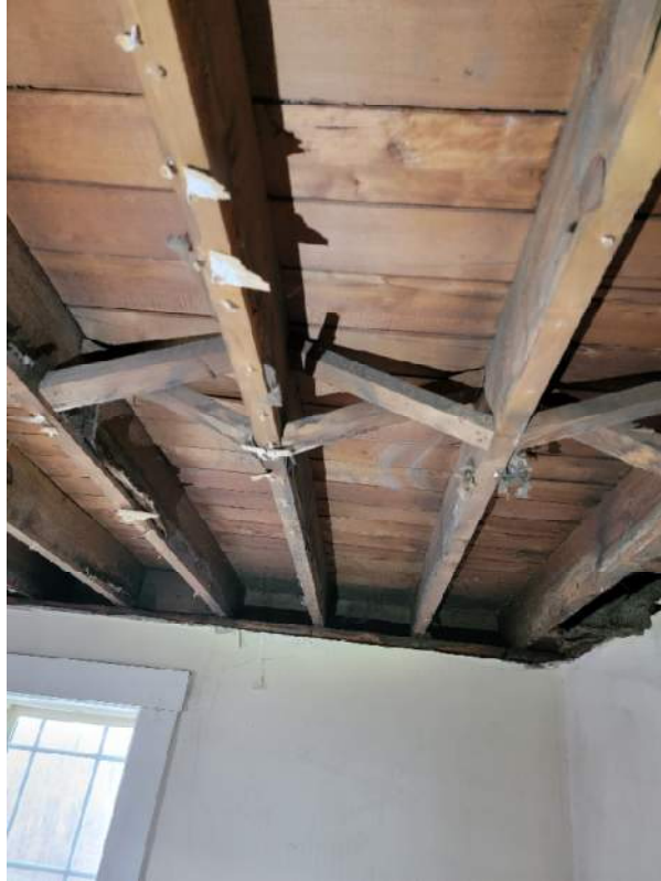
Joists showing nail pull over and nail withdrawal.
